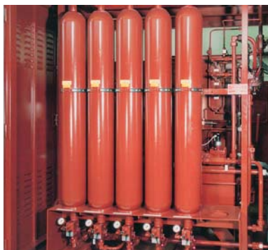
Accumulator Station for presses and test stands.
