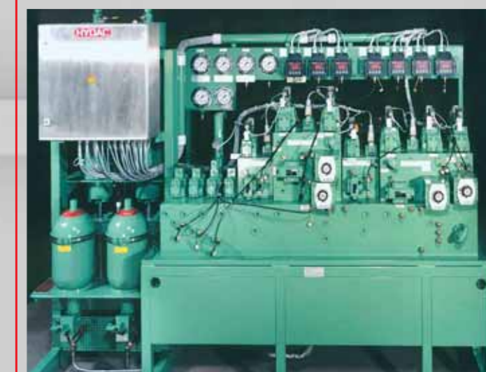
Valve Station for continuous slab casting plant.
