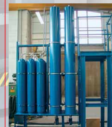
Piston Accumulator Station with back-up N 2 bottles, e.g.: electric oven safety function.
