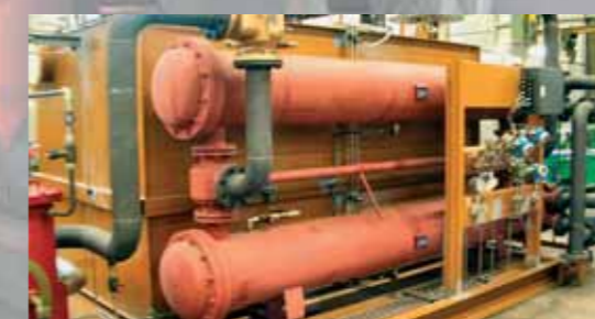
Blast Furnace Gas Expansion Turbine, oil tank volume 9,500 l, power 500 kW, flow rate 760 l/min.
