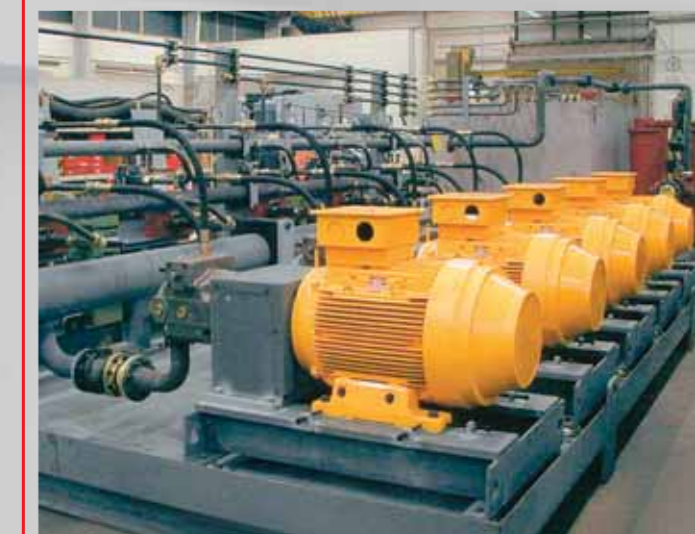
For example: Pump Station for Strip-Winding Plant, oil tank volume 6,000 l, driving power 575 kW, flow rate 1,900 l/min.
