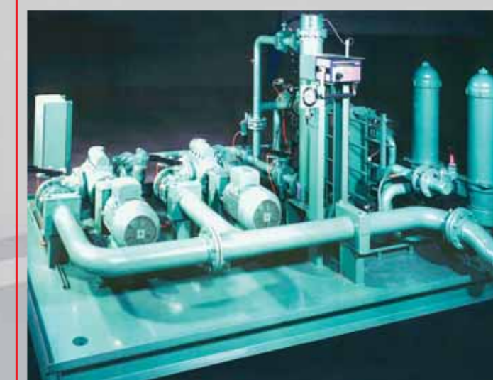
Bypass Heating Filter Cooling Circuit for continuous casting plant.
