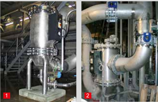
Fig. 1: Application: In the waste water treatment plant of a paper factory, waste water is treated in a ozonisation stage. Disruption is caused by plastic particles carried over from waste paper treatment.
