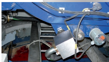
Drain valve for gearbox
