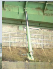
Cylinder for water control sluice gate
