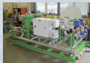
Cooling and seal water treatment
