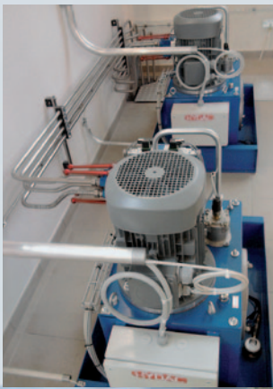
Power unit for weir wickets
