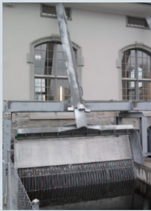
Cylinder for trash rack cleaner
