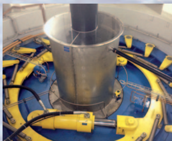
Hydraulic cylinder (servo motor) Turbine control guide vane adjustment
