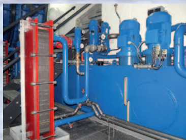
Water cooling and filtration system (bearing oil)
