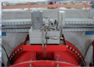
Power unit for butterfly valve control
